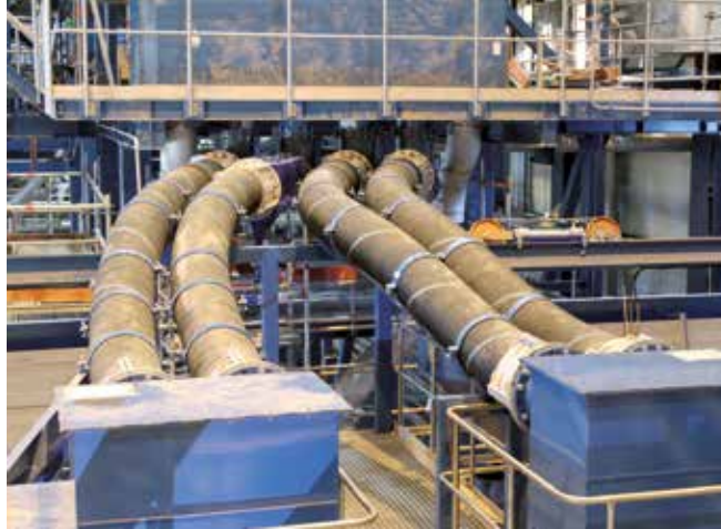
Slurry hoses systems
