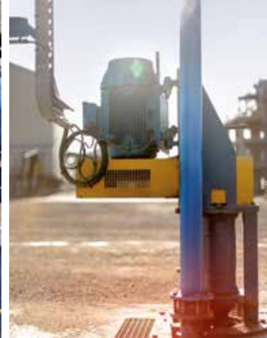
Vertical slurry pumps
